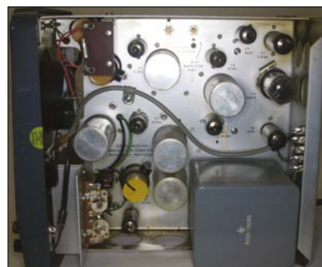
Figure 4. Capacitor leakage and overheating.
