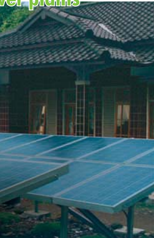
Standalone solar power installations play a vital role in regions lacking significant electrical infrastructure. This is a 4.2 kW setup in Indonesia (photo: Schott Solar GmbH).
