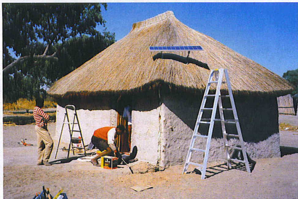
Figure 1. An isolated solar panel system gives a degree of independence from the mains. (photo: Phocos)
