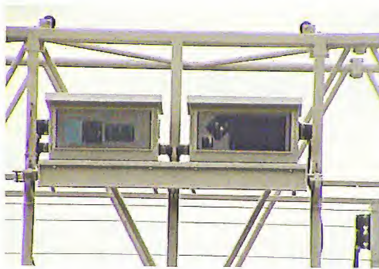
The existing motorway gantries fitted with vehicle recognition sensors for toll collection. (Picture: Toll Collect)
