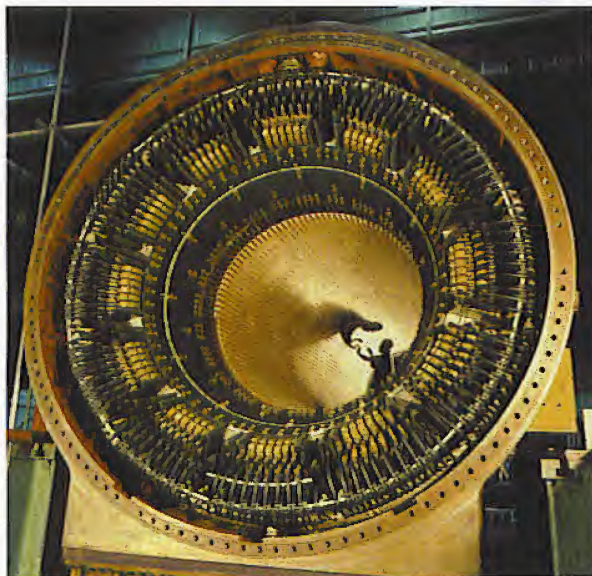
Figure 6. Temperature measurement using fibre-optic sensors inside a 1300-MW generator with extremely high electrical and magnetic field strengths. (Photo: Siemens)
