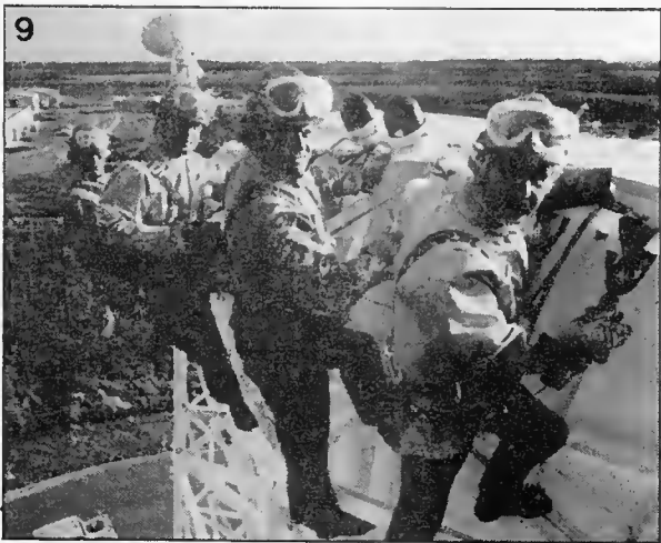
Fig. 9. The antennas are painted regularly: each one takes a 1000 gallons of marine paint and two full seasons' painting. Photograph courtesy of British Telecom.
